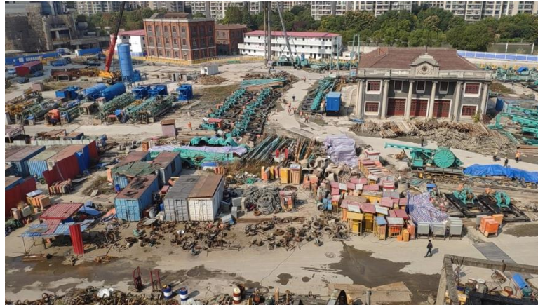
Figure 5: Workers on the way to their lunch break on the construction site of the ‘1000 Trees’ project by Heatherwick Studio, Shanghai, November 2019. Photograph by C. Westermann.
